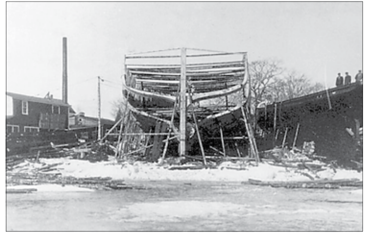
The four-master vessel Arthur H. Zwicker is under construction in this 1918 photo. The boat was captained by Walter Creaser.
